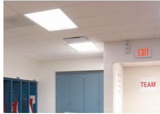
Exit and Emergency
