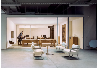
Connected lighting systems
